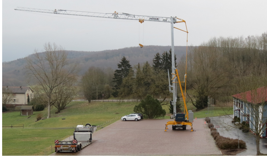
Figure 1: The brand new HUP M 28-22 crane by Potain/Manitowoc. Self-erecting cranes, like the Hup, are transported by truck (the trailer is visible on the picture) and then rapidly erected through “automatic unfolding” of the structure. They are 10 to 30 meters high and are operated from the ground through remote control. Image courtesy of Manitowoc.
