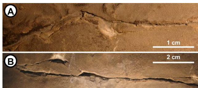
232 233 Figure 6 – Irregular and chipped pattern of natural fractures on floor of upper gallery (in 234 between basins B1 and B3). Pictures Fantine Bellanger/PCR ARBap.
