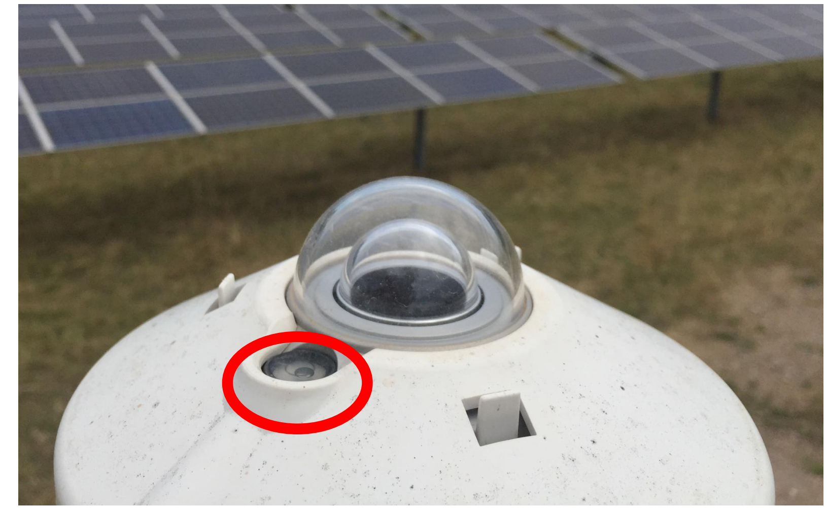
Example of misaligned horizontal pyranometer for PV plant monitoring
