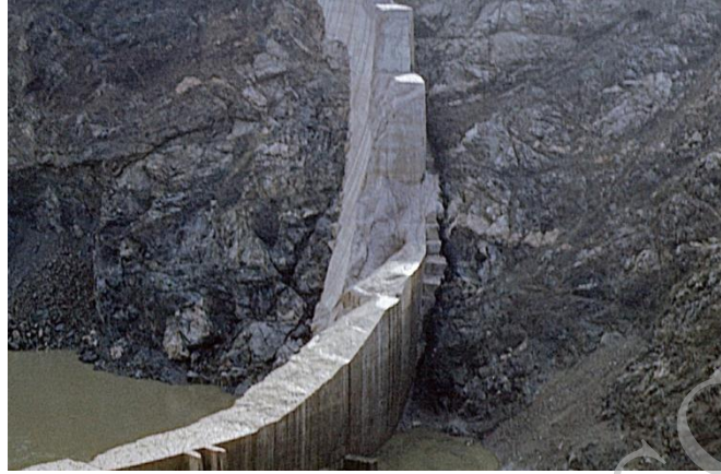
Fig. 8. A conspicuous open crevice separates the dam concrete from the rock mass upstream (photo J. Duffaut , Dec. 20, 1959)
