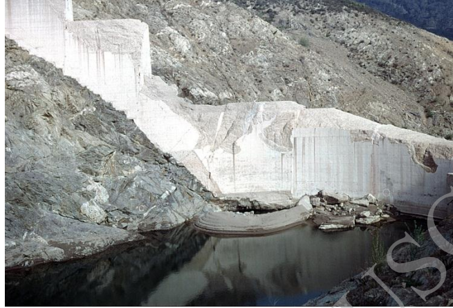
Fig. 12. The debris sill built under water by the flow below cantilever FG (photo P. Duffaut, May 1960).
