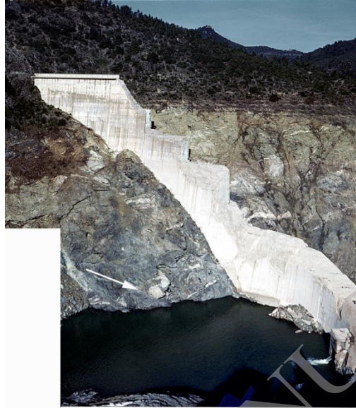
Fig. 6. Remains of the dam on right valley side and valley bottom; the rock appears crisscrossed with white pegmatite dykes; the arrow shows the main fault; the river flow passes through the outlet valve (two assembled photos, J. Duffaut, Dec.20, 1959)
