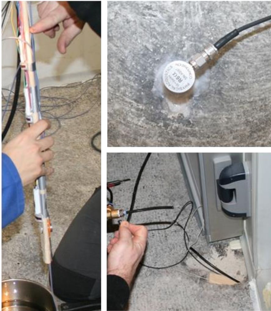
Fig. 3. Central multi-sensor ultrasonic probe being placed in the borehole (left), ultrasonic sensor fitted on the surface (top right) and ultrasonic probe shifted in place (bottom right).
