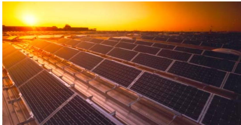
Fig. 1.18: General overview of the Munich Trade Fair Centre roof integrated PV system (Courtesy of Solarenergieförderverein Bayern e.V.).
