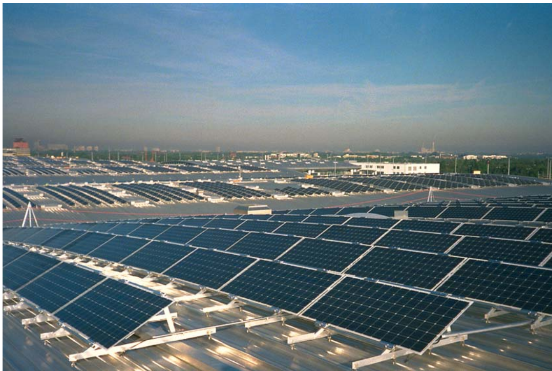
Fig. 2.9: General overview of the Munich Trade Fair Centre roof integrated PV system (Courtesy of Solarenergiefördereverein Bayern e.V.).
